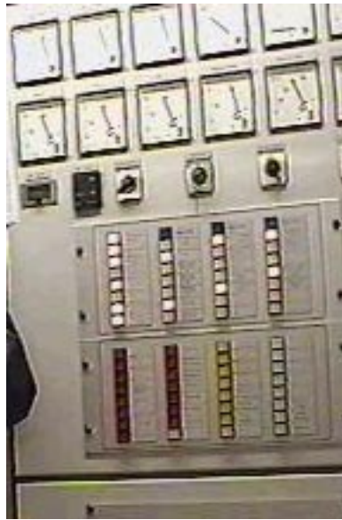
Fig 4: The meter panels
